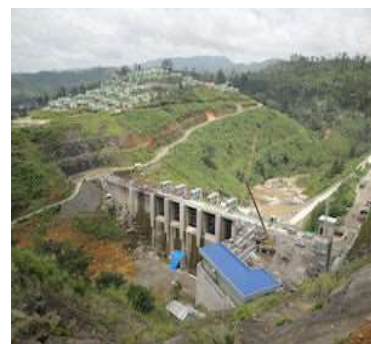
Img 2.4.10 Bank-side Reservoir
