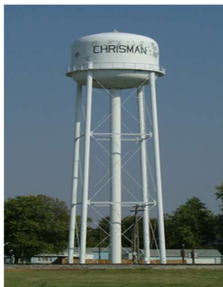
Img 2.4.11 Service Reservoir
