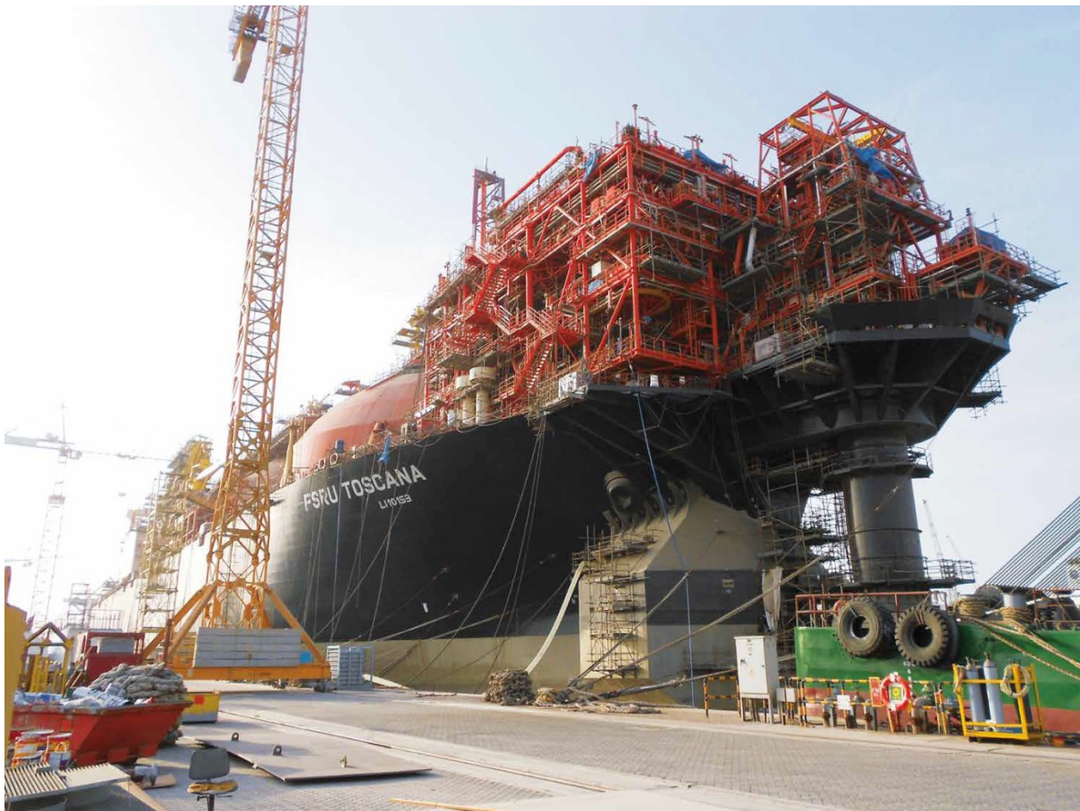
Picture 17: Construction of regasification section by Saipem SA at FSRU Toscana [48, p. 53]
