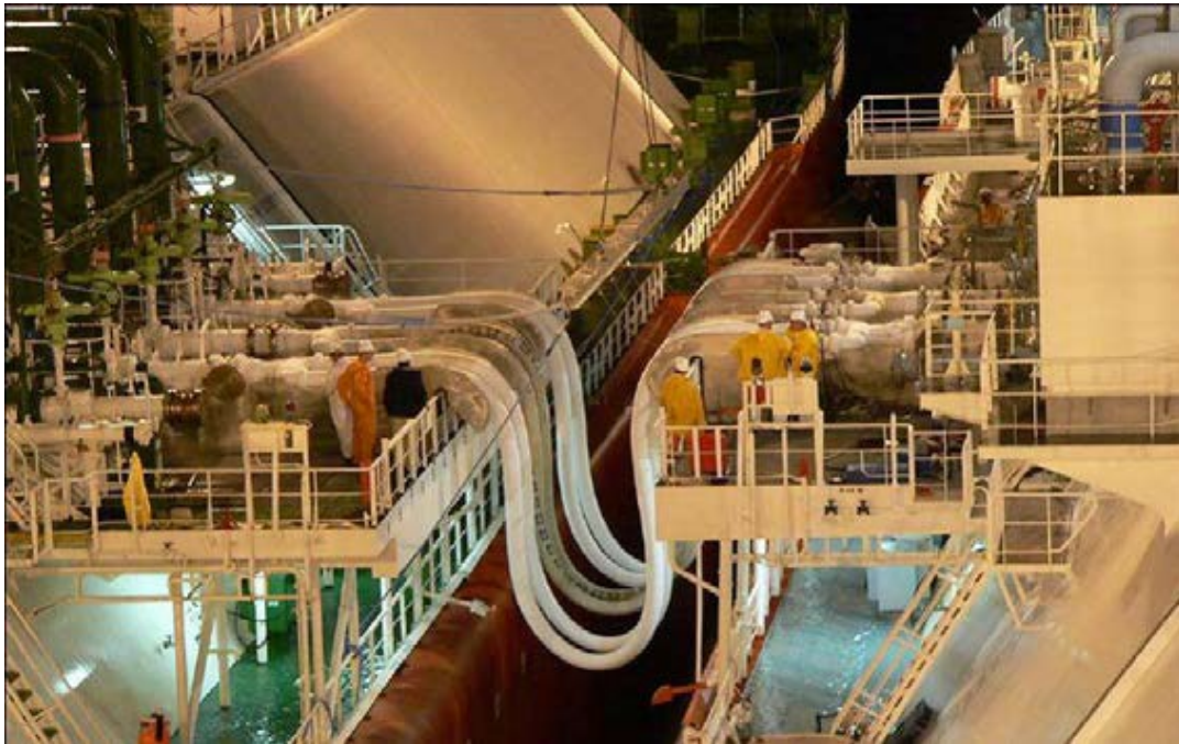
Picture 13: LNG transfer side by side using flexible hoses [31]
