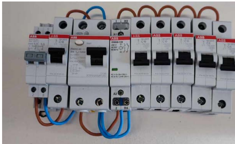
Figure 54: Electrical Control Panel Circuit
