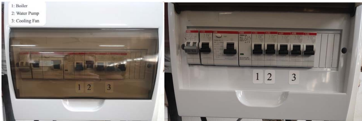
Figure 53: Stickers of Electrical Control Panel Instructions
