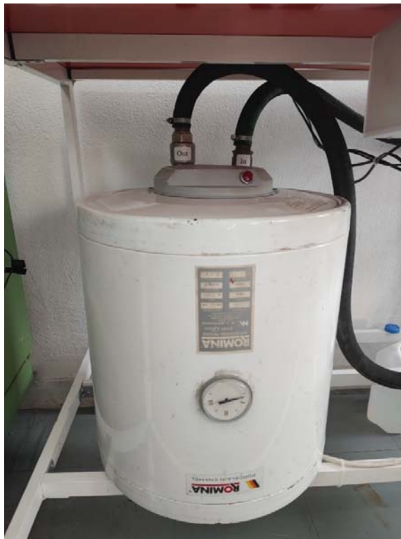
Figure 35: Boiler – Water Heater (Romina)
