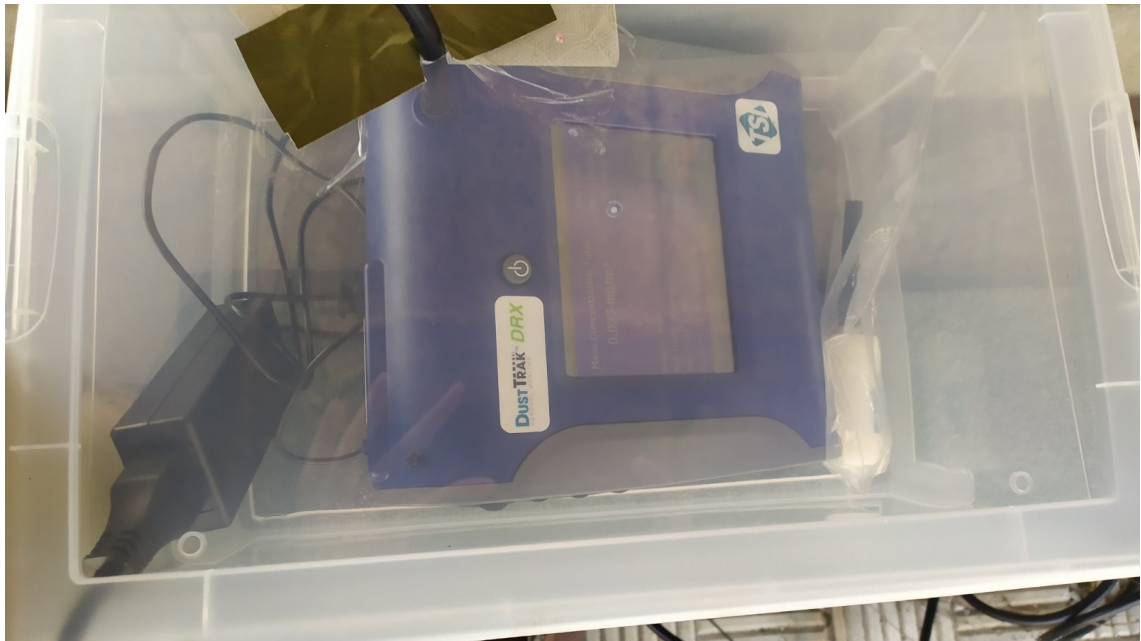
Illustration 30: TSI DusTrax devices installed.
