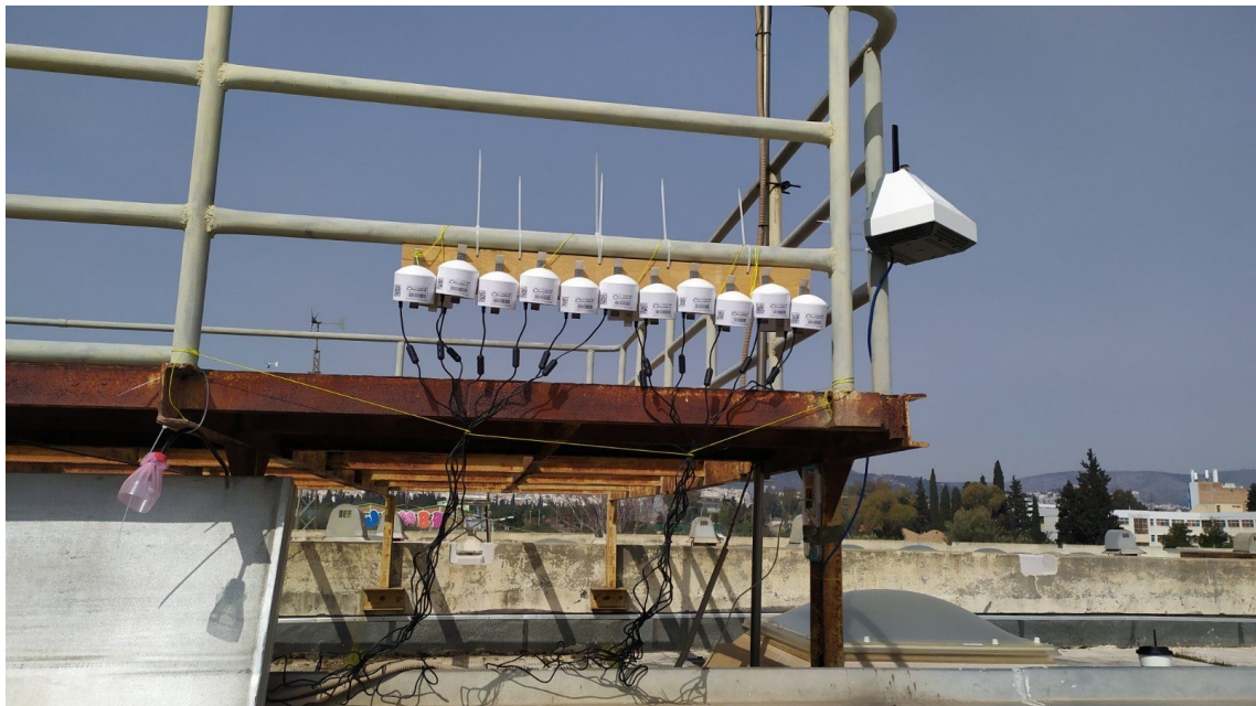
Illustration 29: Purple Air and AQ Mesh devices installed.
