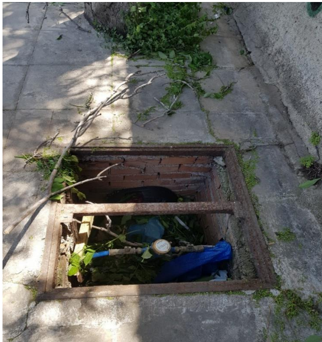
Image 95 Open manhole at Petrou Ralli Street, 2022
