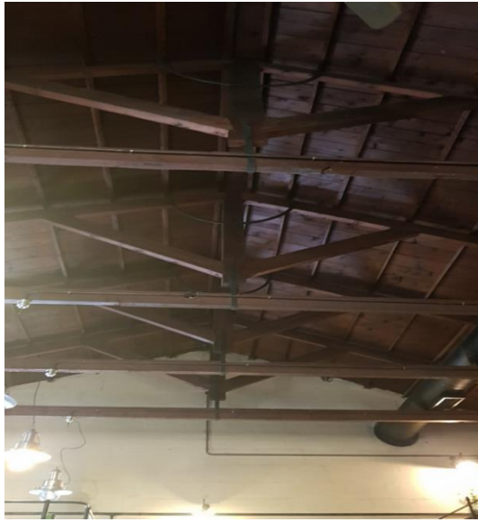
Image 127 Wood ceiling of the A.E.X.B. power-generating facilities, 2019
