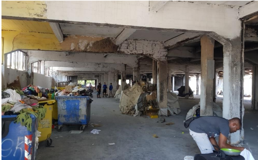
Image 44 Industrial building at Kastorias Street, part of the wastepicker market in the Eleonas that sustained fire damage, 2022
