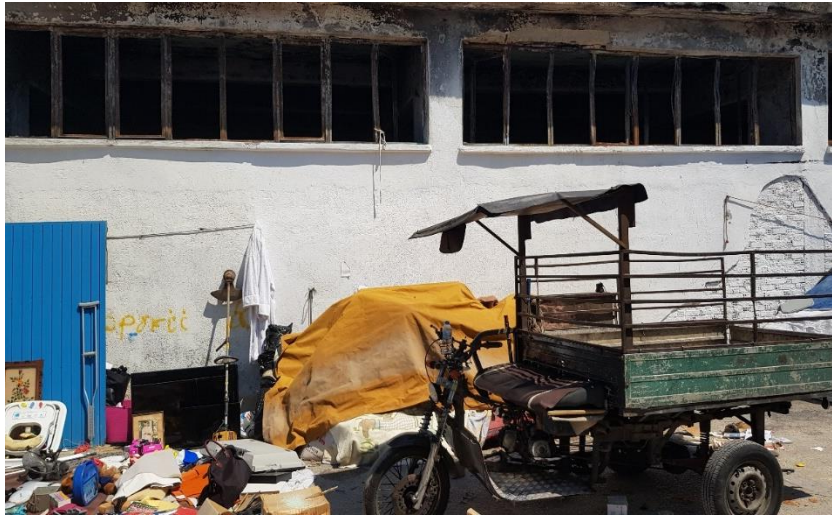
Image 50 Industrial building at Kastorias Street, part of the wastepicker market in the Eleonas that sustained fire damage, 2022
