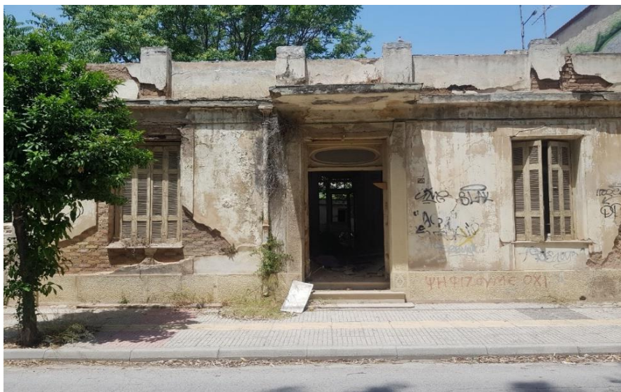
Image 35 Abandoned residence at 2 Estavromenos Street, 2022
