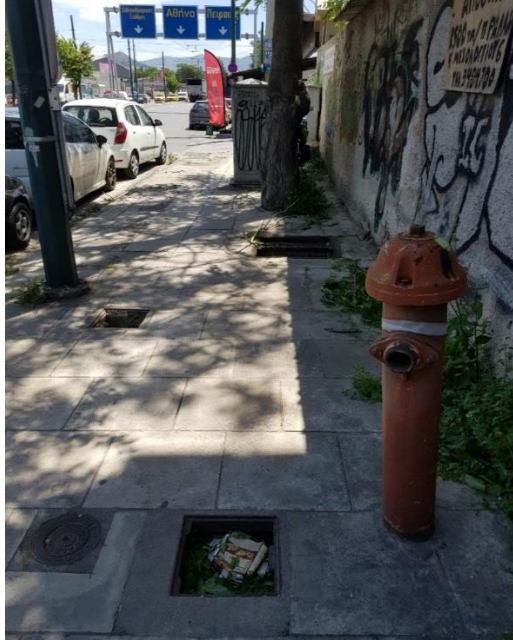
Image 94 Open manholes at Petrou Ralli Street next to the corner at Aristotelous Street, 2022
