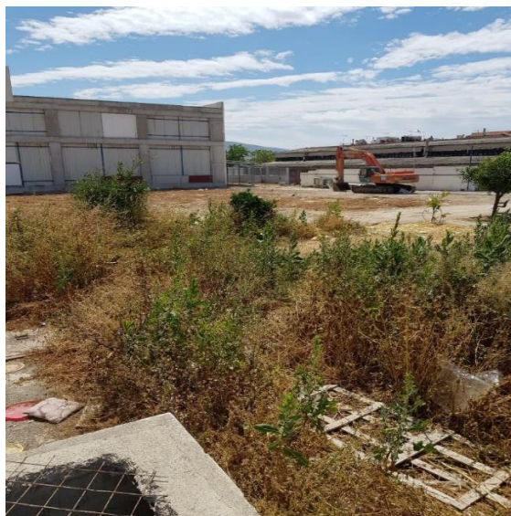
Image 87 Demolition of industrial structures at the former V.I.E.R. site at Doridos Street, 2022
