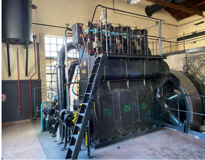
Image 123 Power-generating facilities of A.E.X.B., 2019
