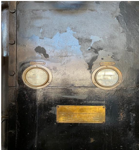
Image 124 Power-generating facilities of A.E.X.B. DIESEL MAN engine, 2019
