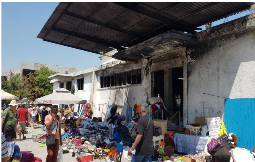
Image 45 Industrial building at Kastorias Street, part of the wastepicker market in the Eleonas that sustained fire damage, 2022
