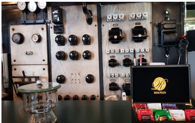
Image 128 Power-generating facilities of A.E.X.B., 2019
