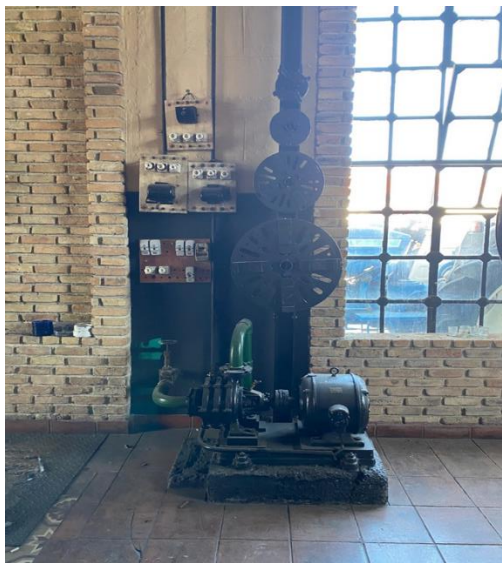
Image 126 Power-generating facilities of A.E.X.B., 2019
